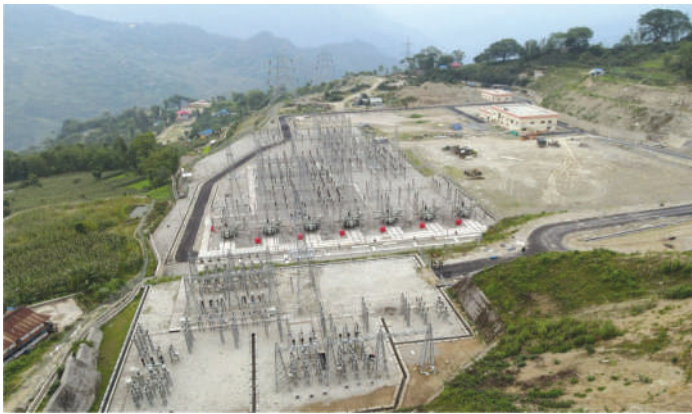
KC-3 Dhungesanghu Substation
