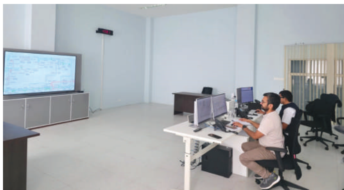
Emergency Control Center (ECC) at Hetauda
