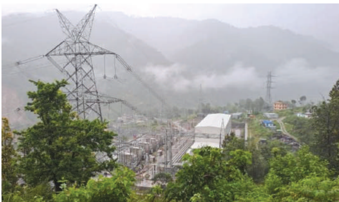
400kV GIS Building and Transformer Banks at 400/220kV 630MVA New Khimti Substation
