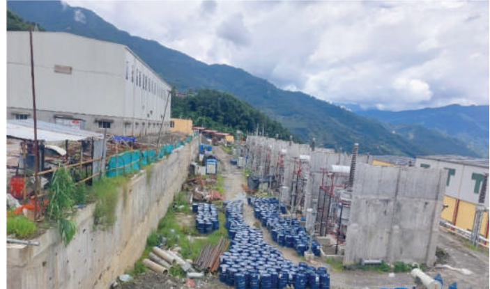
Oil Filtration & Filling works for Transformer & Reactor at 400/220kV 320MVA-50MVA Barhabise Substation
