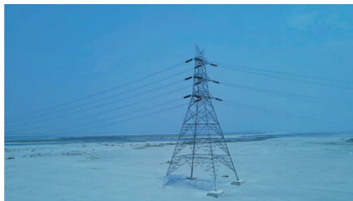
400kV Tower at Koshi River
