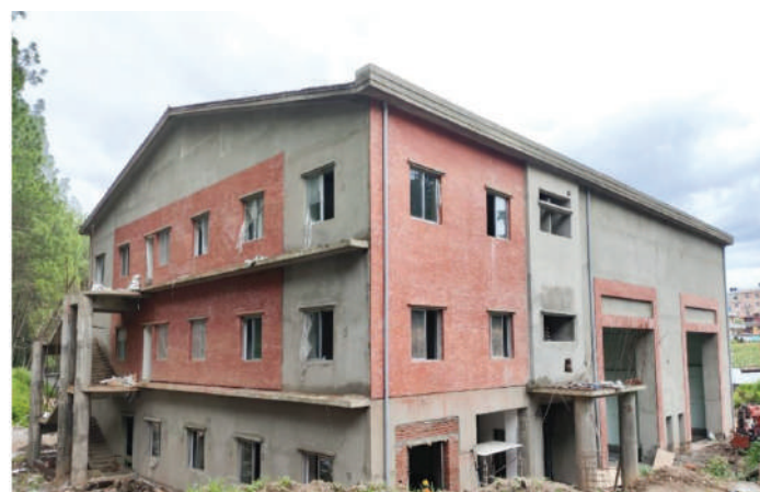
Chovar Control Room Building cum GIS and Transformer Hall
