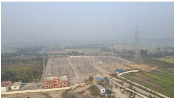
New Butwal Substation
