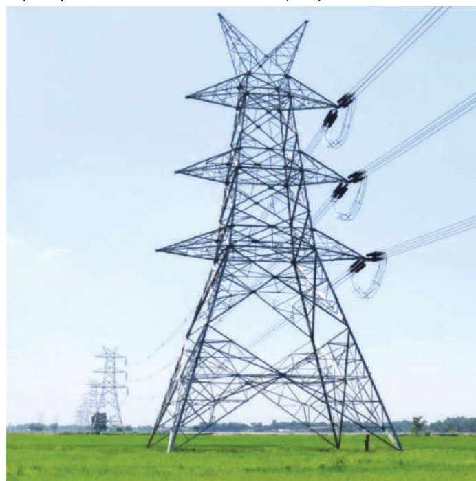
KC-1 Transmission Line (Quad Section)
