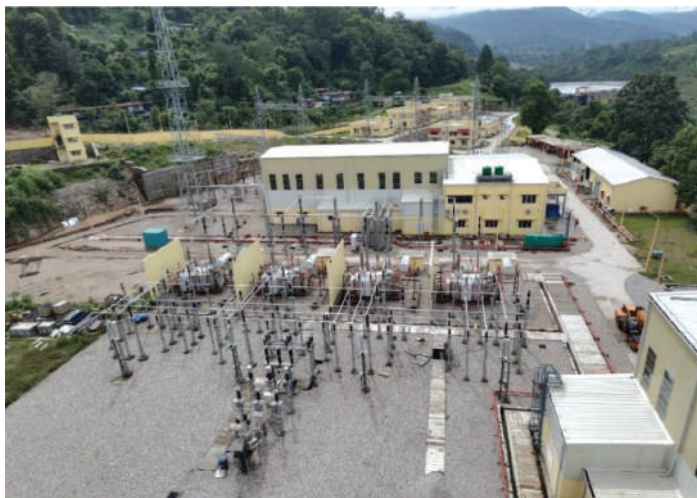
Transformer bank of 1-ph 53.33 MVA transformers in the Udipur Substation, Lamjung
