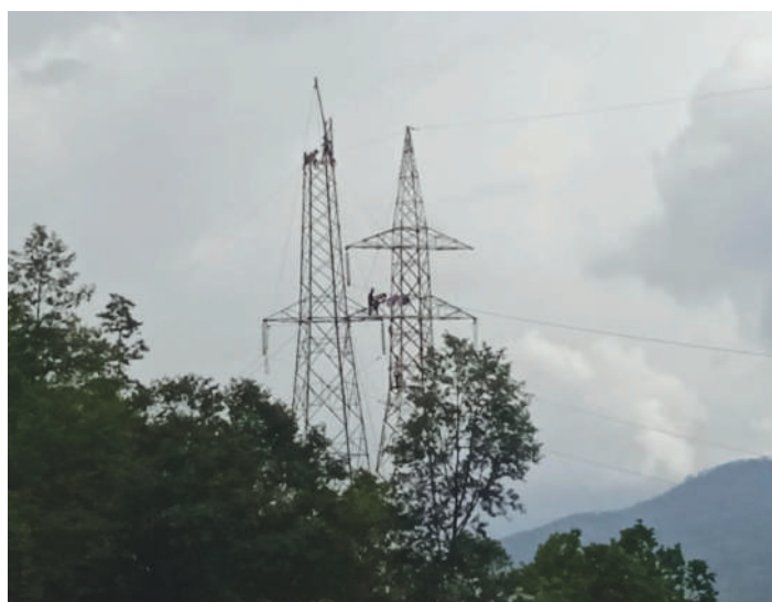
Tower erection and conductor dismantling works at Tower No 59 of Khimti Lamosanghu 132 kV Transmission Line
