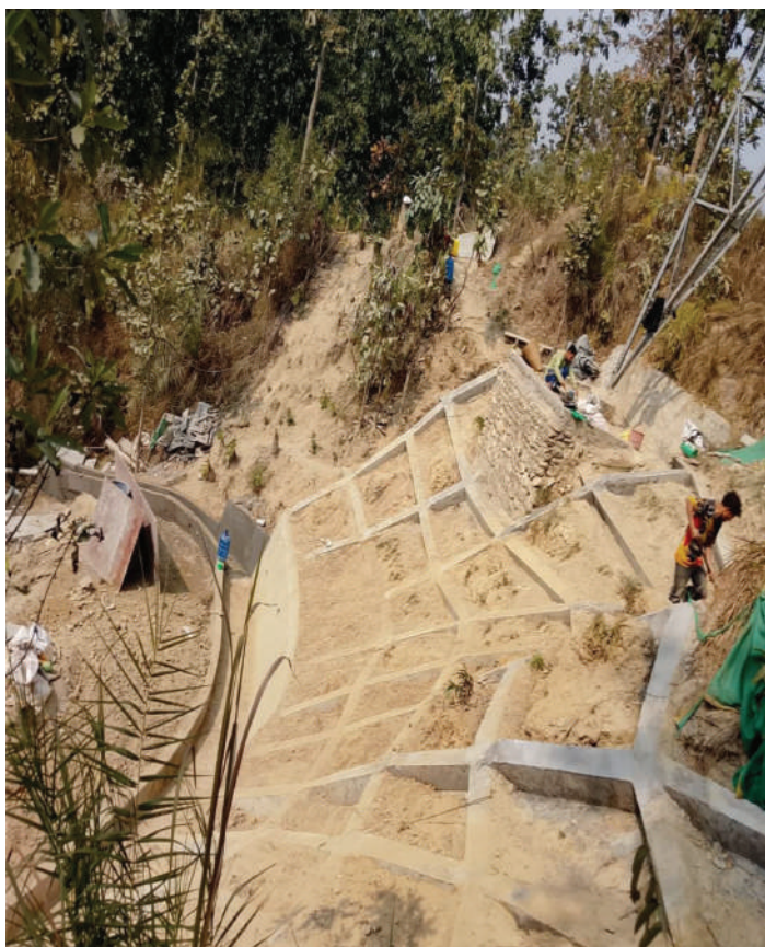
Permanent Protection Works for Tower no 122 and 137 of Khimti-Dhalkebar 220 KV Transmission Line.
