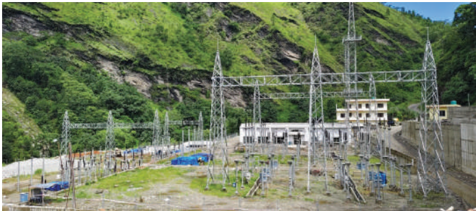
132kV Switchyard with CR Building, Dadakhet Substation
