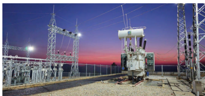
Tamghas 132/33/11 kV Substation
