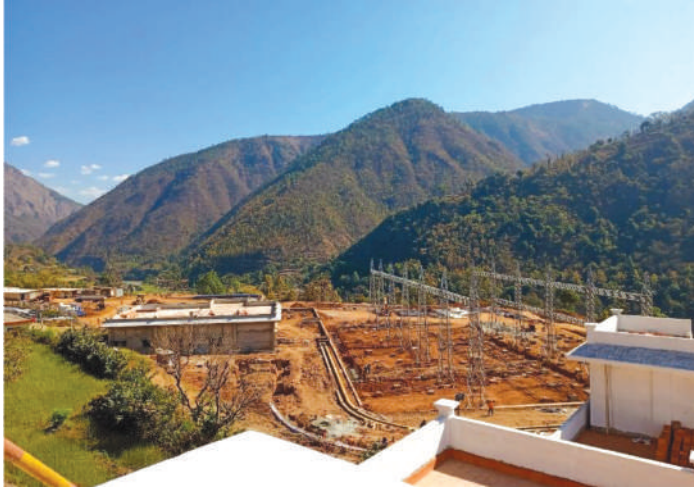
Overall View of Khungri Substation
