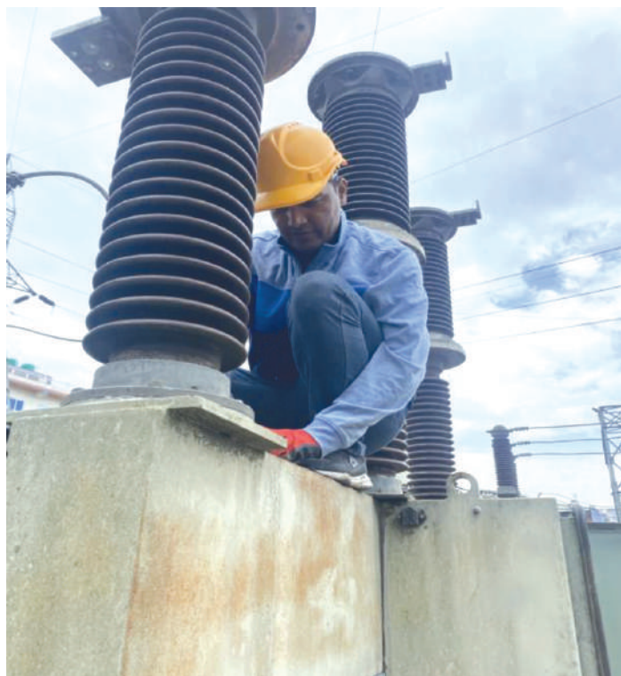
66 kV Circuit Breaker for 66/11kV, 22.5MVA Tr-1, Banepa
