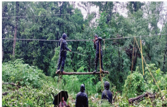
Maintenance of Broken HTLS Conductor of 132 kV Nawalpur-Chapur Transmission Line at Dhalkebar Grid Division
