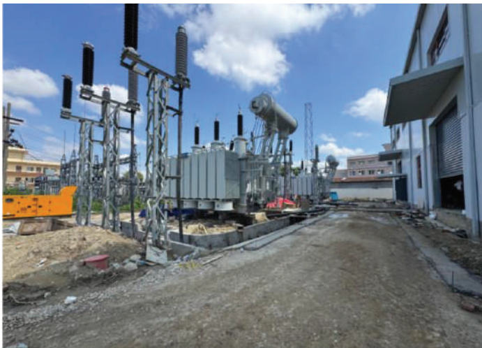
GIS Extension at Birgunj Sub-station
